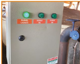
Painel de controle Panel de control
