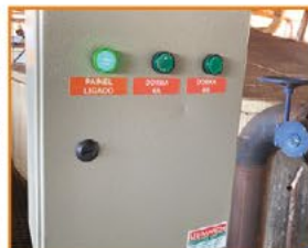
Painel de controle Panel de control
